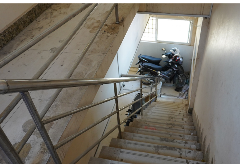
A review of the second floor staircase, showing that a disabled individual cannot access or use the stairs.
